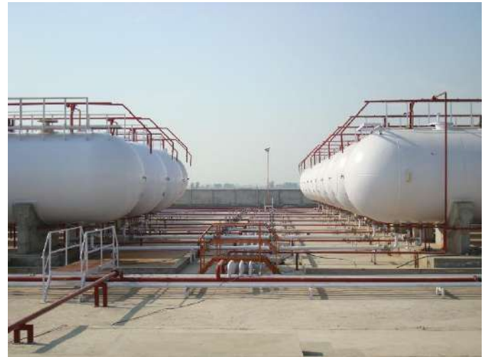
Lub Gas LPG Terminal, Rana Town Lahore (3600 Ton)
