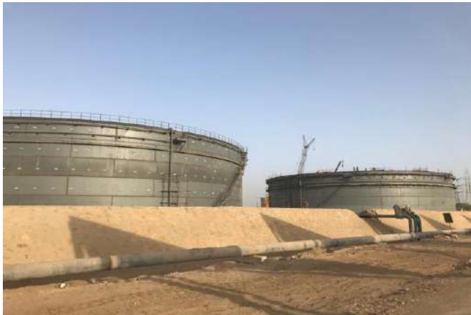
PSO – 02 Nos. 31,000 MT Storage Tanks at Zulfiqarabad Oil Terminal – Port Qasim, Karachi
