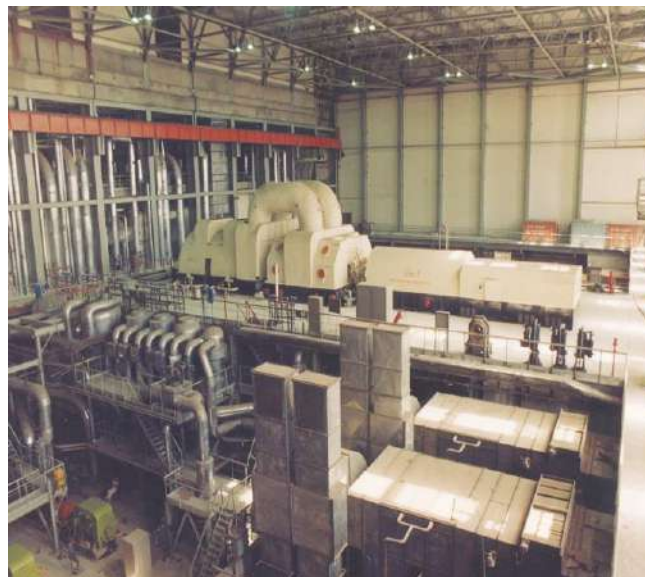
Technopromexport (TPE) – USSR/Russia 3x210 Thermal Power Station - Muzaffargarh
